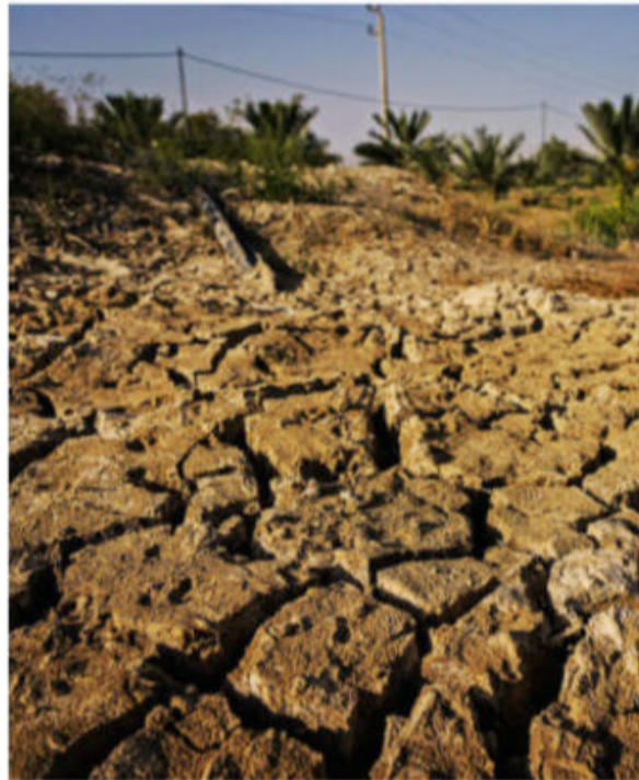
Cracks in the surface
